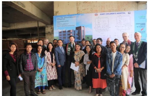
CAP Team and In-patient Unit construction site visit by Hon. Norwegian International Development Minister Mr. Dag-Inge Ulstein.
